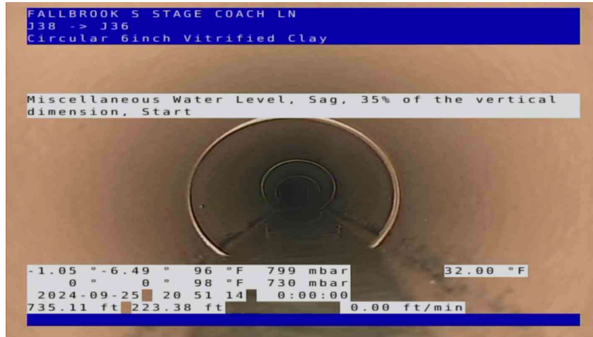
COL-P2PZ-GSMN-J38-J36_948d23d3-3d8b-43a8-9608-af007eb66792_20240925_120241_411.jpg, 00:09:12, 223.38ft Miscellaneous Water Level, Sag, 35% of the vertical dimension, Start
