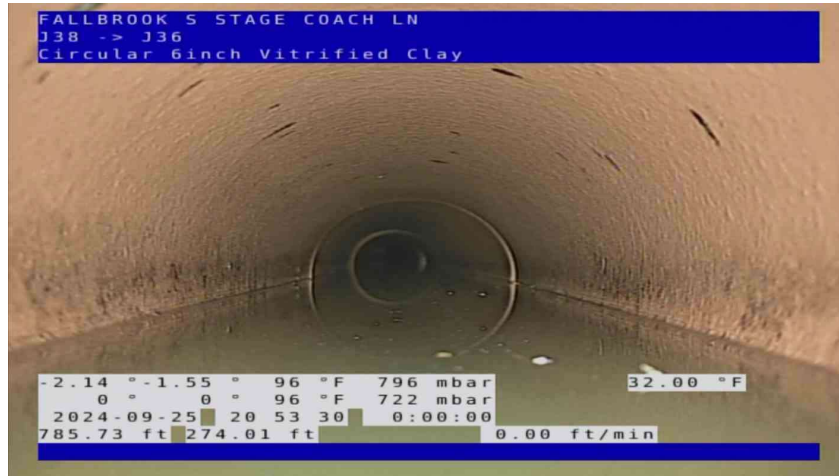
COL-P2PZ-GSMN-J38-J36_658ccc0b-cf2e-4e19-9929-a8dd1c613cf_20240925_120457_540.jpg, 00:10:46, 274.01ft Miscellaneous Water Level, Sag, 50% of the vertical dimension, Start
